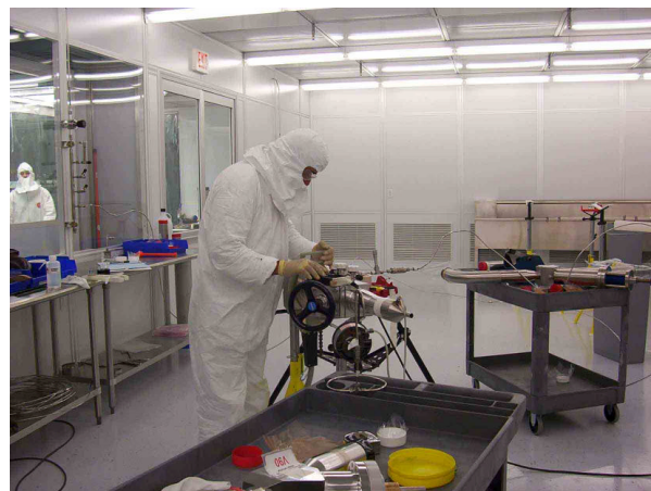
Orbital welding stainless steel tubing for a high purity gas delivery system by a TFS technician
